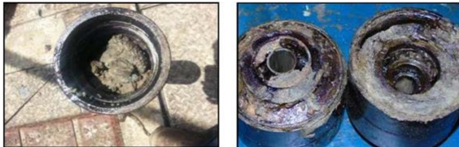
Figure 1.12 Evidence of pump plugging in assembly
